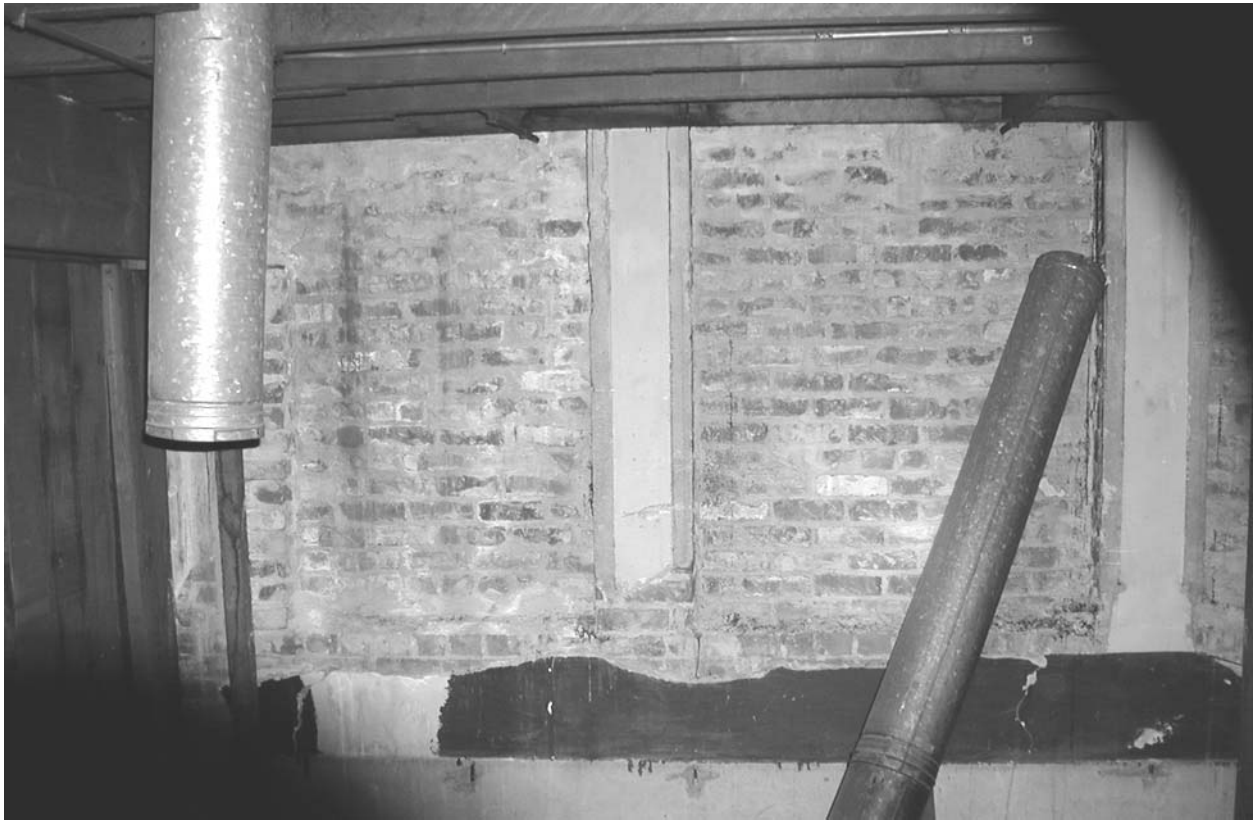
View of upper façade from interior, showing bricked window openings from earlier building / F.Maggi, Oct. 2001
