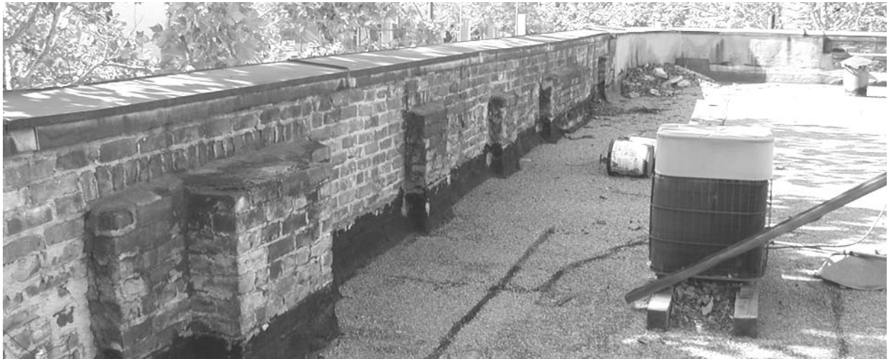
View of parapet of East San Fernando Street wall, viewed from the northeast / F.Maggi, Oct. 2001
